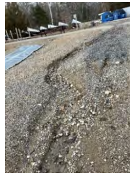
VMB West Lot Erosion 2023
