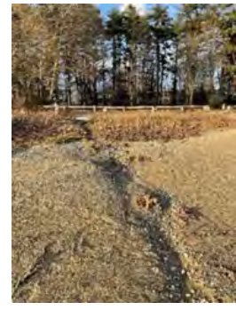
VMB East Lot Erosion 2024
