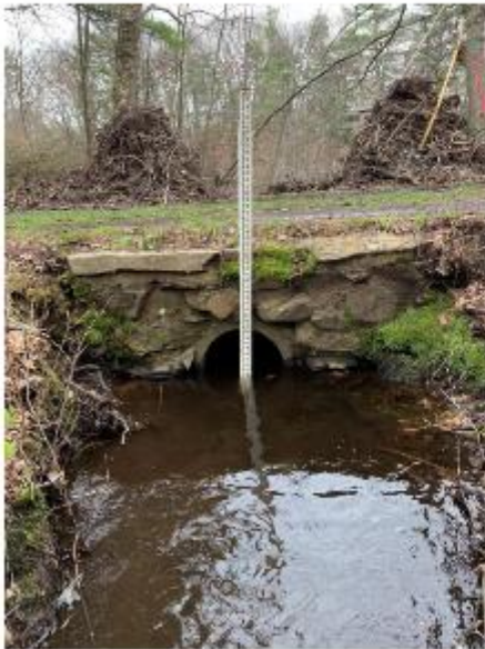
Outlet side of culvert, under cart path. Note piles of debris on both sides of culvert inlet.
