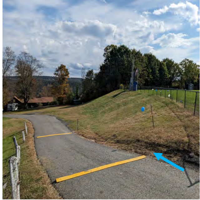
Photo 12-2: Shoulder erosion along the paved access roadway.
