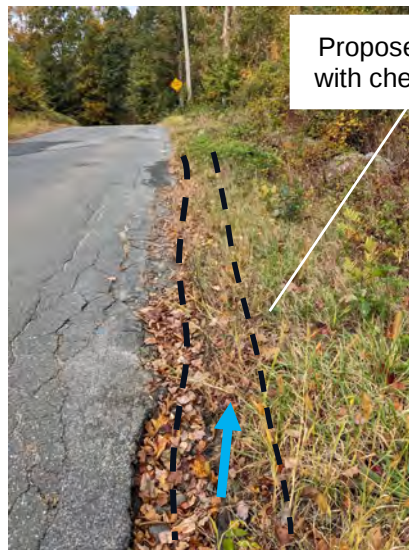
Photo 9-2: Erosion along the shoulder of Carpenter Road.
