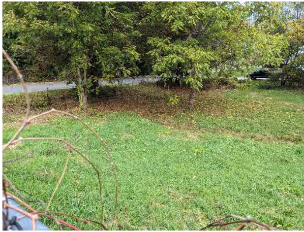
Photo 10-1: Outlet for drainage system on Carpenter Road.
